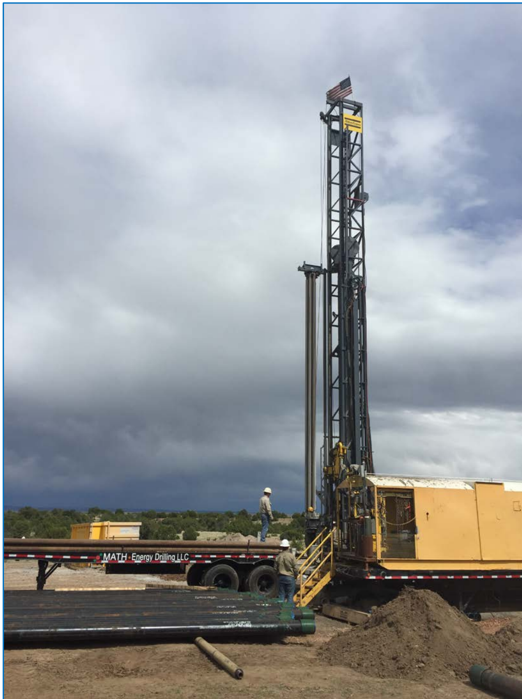
Austin's COO, Mr. Tm Hart at the controls of the Math Energy Drilling Atlas Copco RD 20 Range 3 Drill Rig
