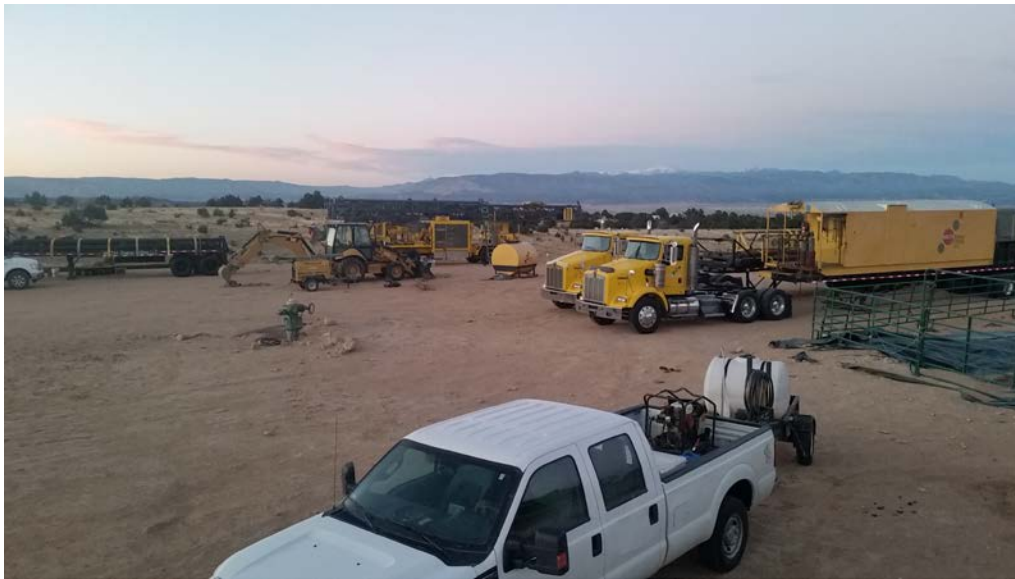
Site preparations at the C18#2 well are almost complete with 90% of equipment in place
