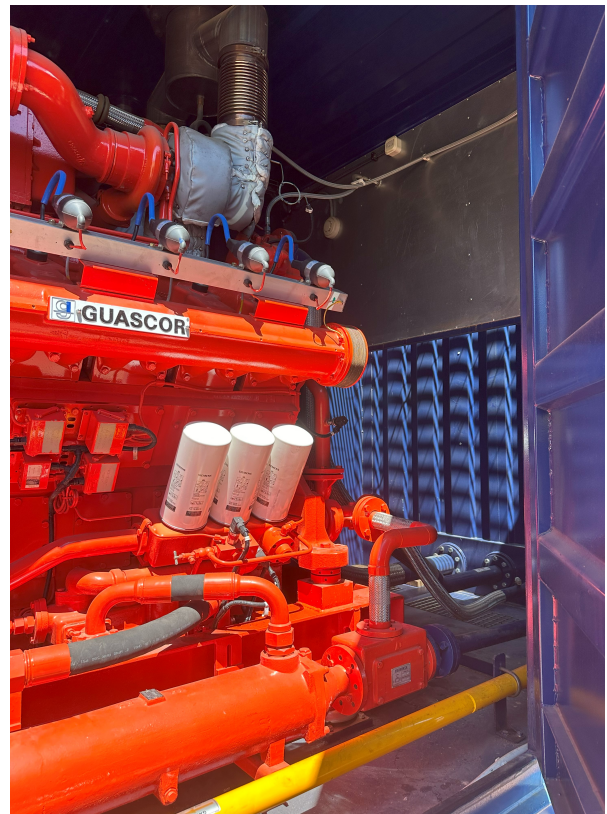
Gas-Fired Genset Internal View
