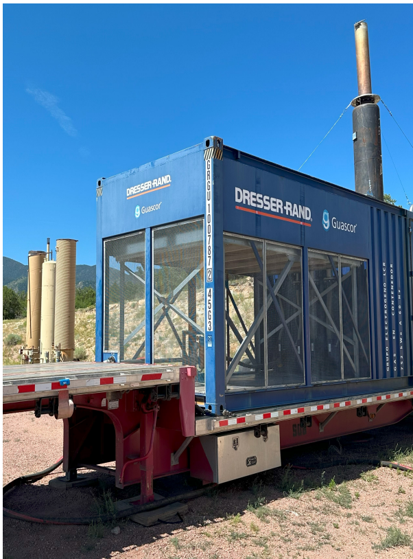
First of two Gas-Fired Generators on-site at Pathfinder Well
