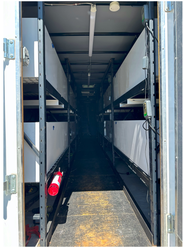
On-site Data Centre Module Interior
