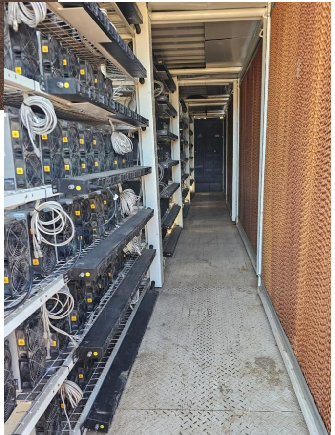
INSTALLATION OF MINERS WITHIN MDC
