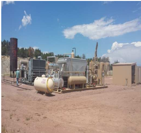
Pathfinder Gas Processing Plant
