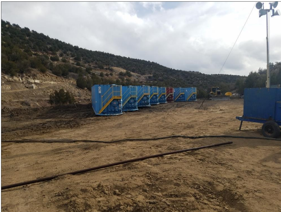
Figure 2: Several frac tanks in place for fracture stimulation operations.
