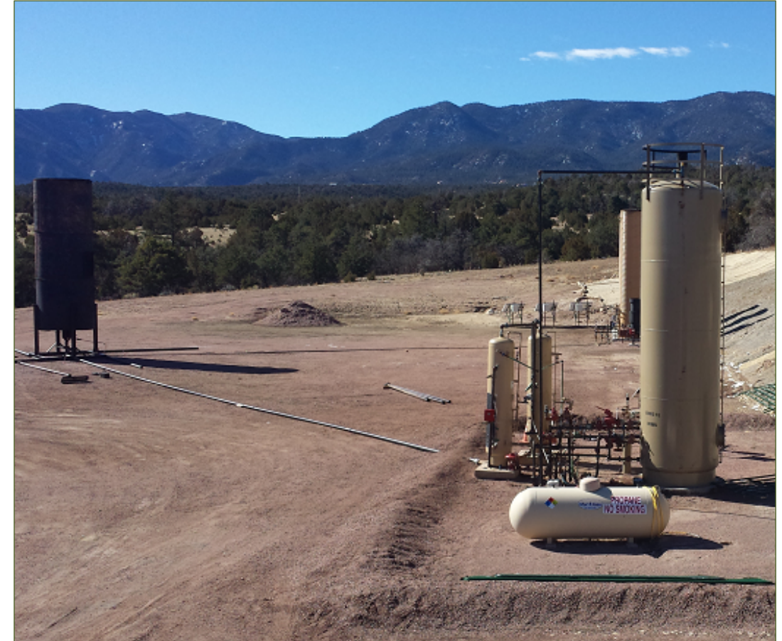
Oil/Gas Separators Installed At Pathfinder For Higher Gas Volumes
