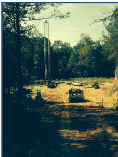
WORK-OVER RIG INSTALLING THE INJECTION SYSTEM IN THE BOARD OF EDUCATION SALT WATER DISPOSAL WELL
