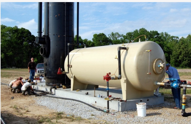
Oil and Water Separation Facility
