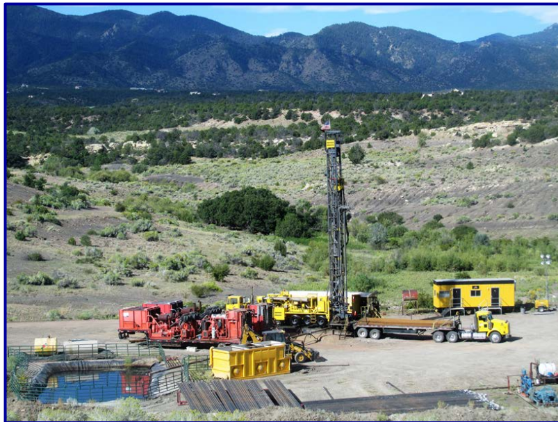
The Atlas Copco RD20 range 3 drill rig and equipment at the Columbus #1 Well site
