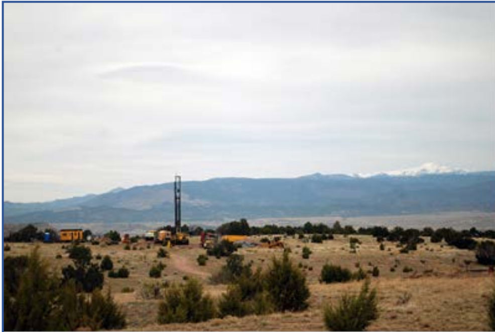
Operations underway at Austin's 15,282 acre flagship Pathfinder project in Fremont County, Colorado
