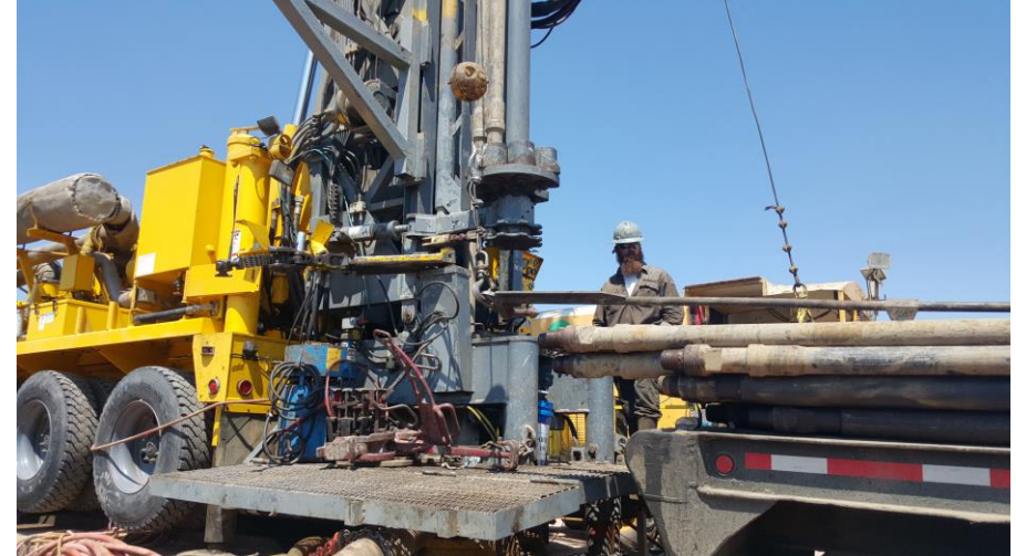
Final Rig preparations are made, and the drill steel is moved in to position
