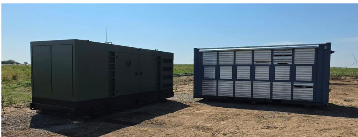
Images 1-3 above: power generation equipment and first third party ASIC container on site at the Charlie #1 well ready for installation mid next week.
