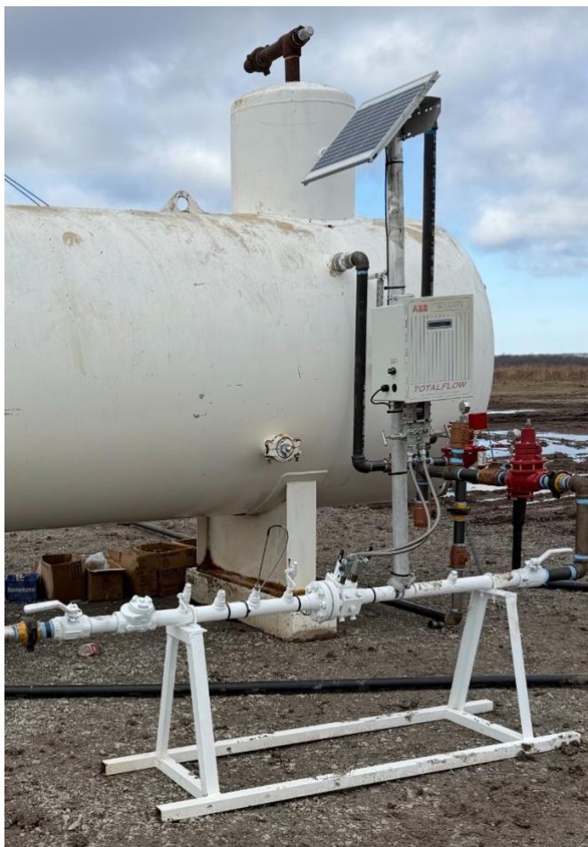
Figure 1: Edwards Lease Gas Separator Installed
